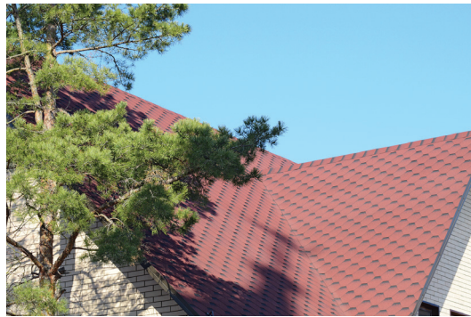
Tree branches too close to roof
